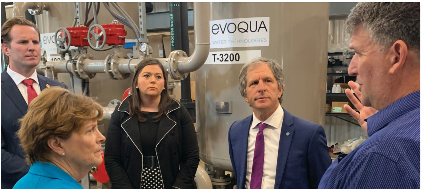
EPA Region 1 Administrator and PFAS Executive Council co-chair David Cash tours a drinking water treatment facility in Portsmouth, New Hampshire, with Senator Jeanne Shaheen and community leaders.
